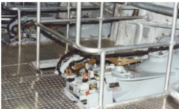
HM571 Jet Installation in Mr Mel
